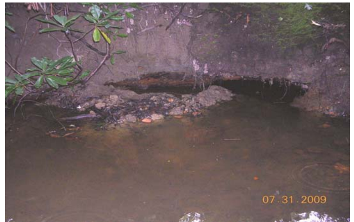
Undercut Bank Due To Dredge Operation
