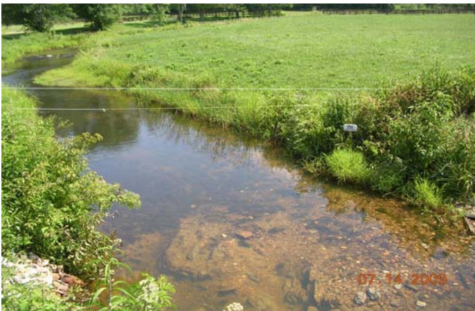
Disruption of Substrate Due to Dredging (note vegetative cover upstream)
